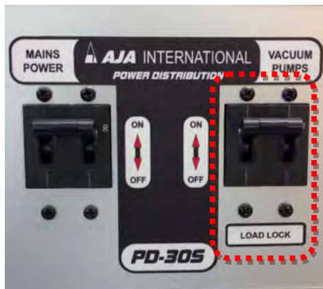
Figure 1 Loadlock pump control
